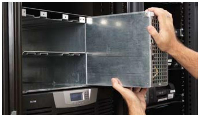
IT staff can easily install electronics modules
